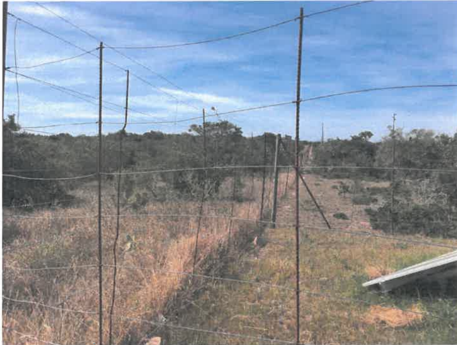
Figure 4: An example of the perimeter fence line which requires repair and maintenance work
