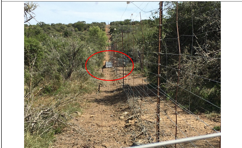
Photo 2-3: An example of an existing gabion structure (circled in red) installed at a low-lying area along the fence line.
