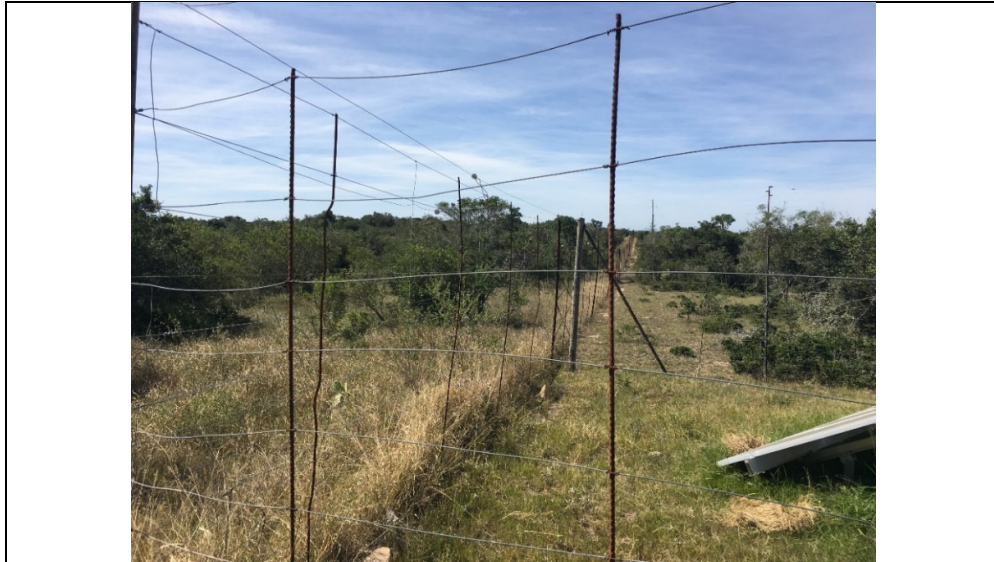
Photo 2-2: An example of the perimeter fence line which requires repair and maintenance work.
